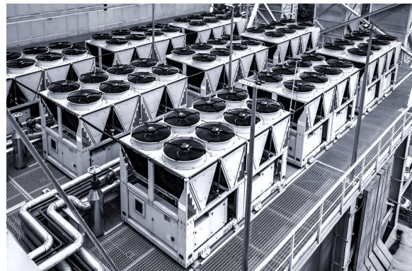
Rooftop air cooling system. Source: Area.
