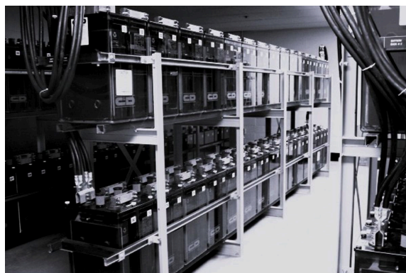
UPS batteries. Source: Kim Otte, 2010.
