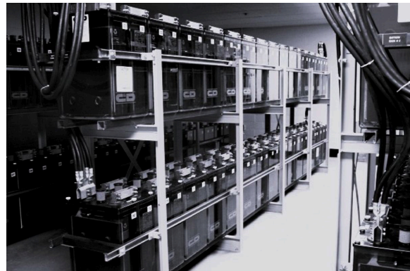
UPS batteries. Source: Kim Otte, 2010.
