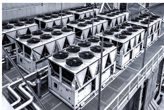
Rooftop air cooling system. Source: Area.
